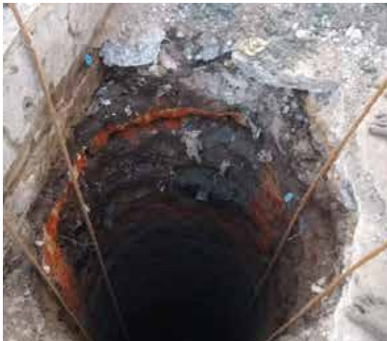
In September 2018, we built 8 rainwater harvesting pits in Mylapore [Chennai] with the technical assistance of Mr Sekar Raghavan of Akash Ganga Trust
